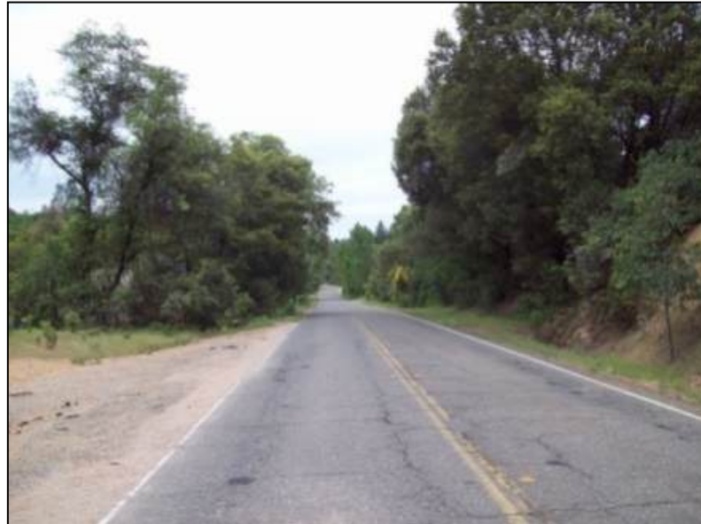
Lake Boulevard north of Highway 151 Note dense brush and trees up to edge of pavement.
