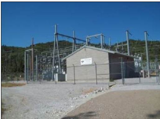
City of Shasta Lake Substation
