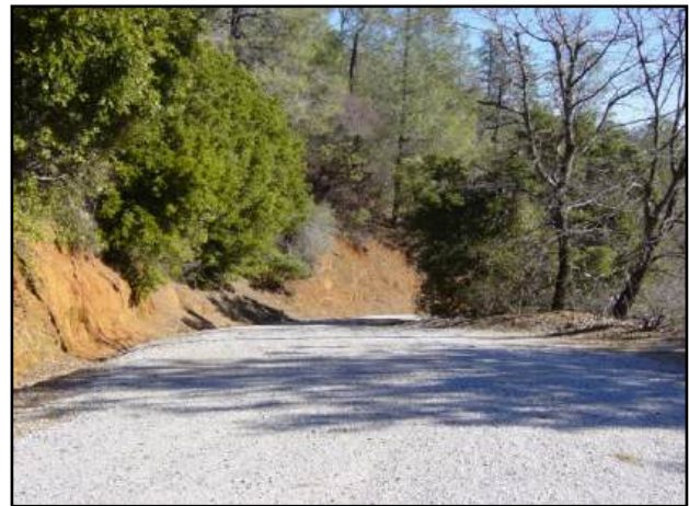
Top of The Hill Road showing brush encroachment
