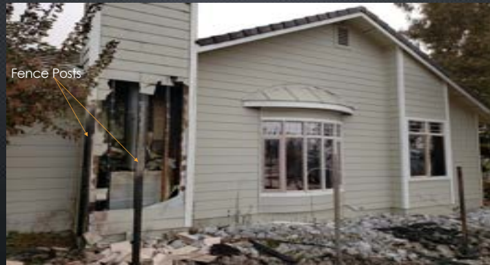
Carr Fire: Wood fence connected to structure. Note: Siding is non-combustible fiber cement (ex. Hardieplank)
