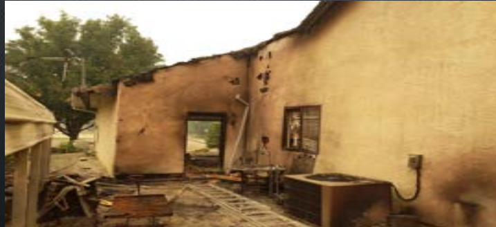
Carr Fire: Exposure to home from trailer igniting, trailer was exposed to vegetation
