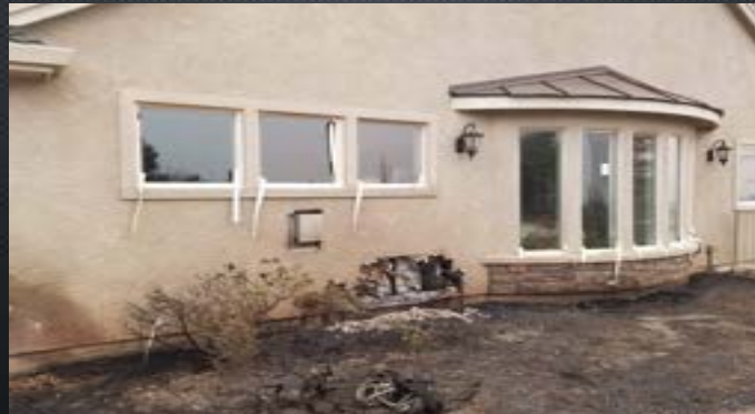
Carr Fire: Wood mulch; home was also exposed to radiant heat *Home was extinguished by neighbor 12 hours after fire front.
